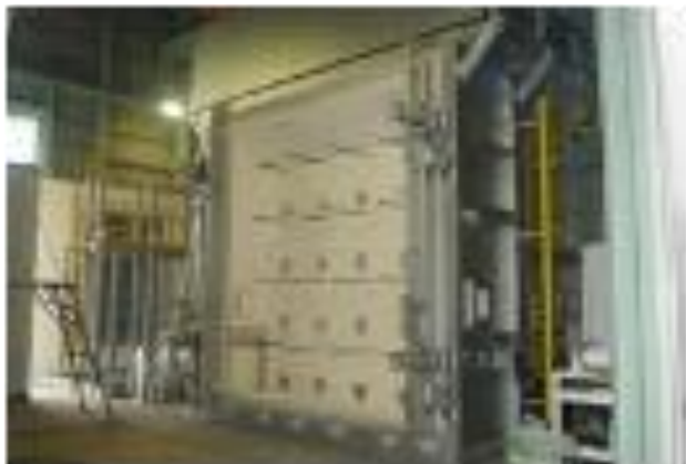
Figure 17: Large wall furnace for façade and window.
