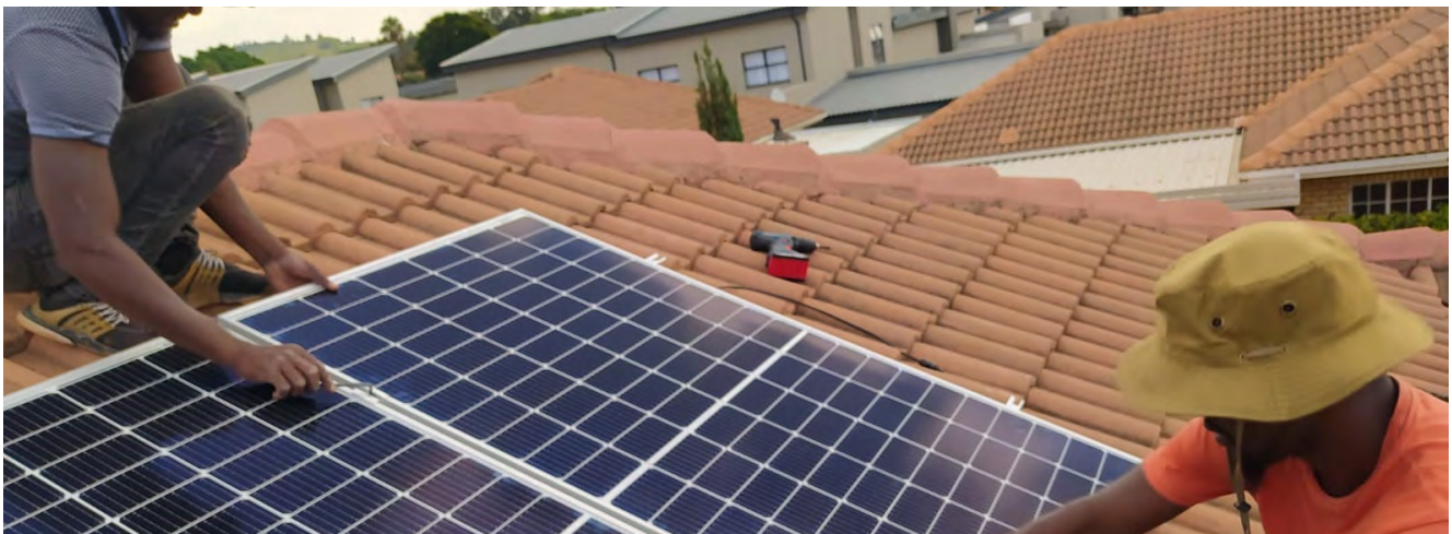
Fig. 68- Residential PV installation during construction in Gauteng Province in South Africa © Dr. Karen Surridge, South African National Energy Development Institute (SANEDI)
