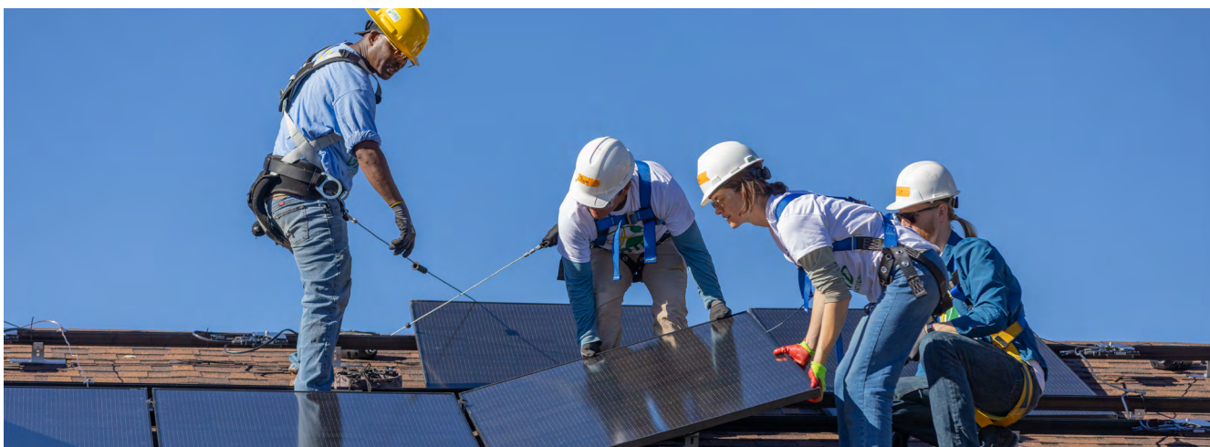
Fig. 75- Staff from the National Renewable Energy Laboratory and GRID Alternatives Colorado install rooftop solar panels during a volunteer event in October 2023. The 6.7 kW solar installation project should provide the home with US$1 200 annual savings over the next 20 years. (Photo by Joe DelNero /NREL)
