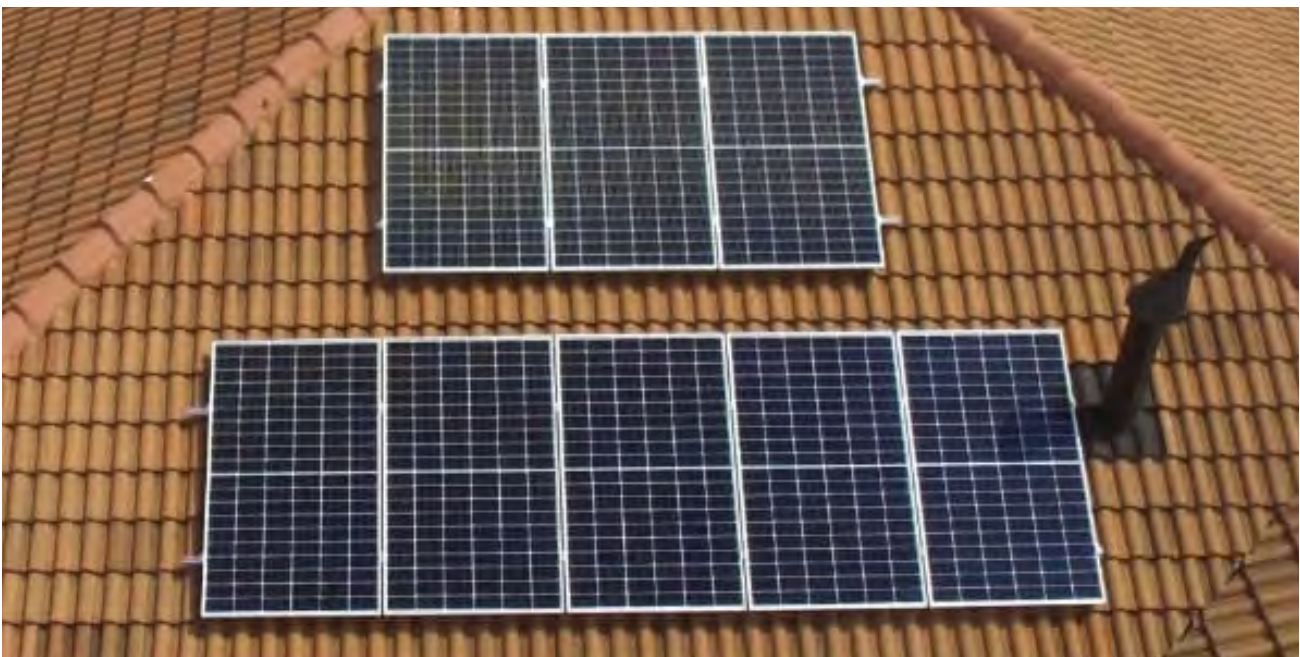
Fig. 69 - Roof-top PV system installation in Gauteng Province in South Africa © Dr. Karen SurrIDGE, South African National Energy Development Institute (SANEDI)
