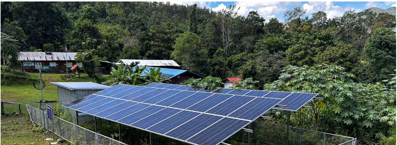
Fig. 74-A centralized mini-grid system with 15 kWp solar panel with 90 kWh BESS installed under the Energy Efficiency and Renewable Energy Support Project for Royal Initiative Projects by DEDE to provide electricity and well-being for distant villagers in Om-Koy district, Chiang Mai.
