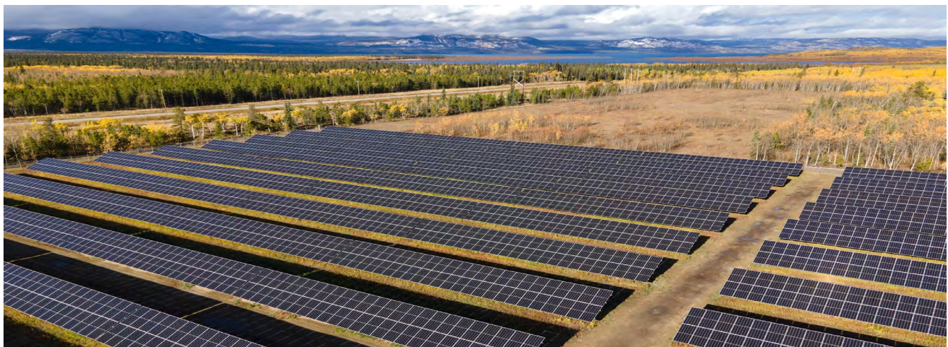
Fig. 34 - The North Klondike grid-tied PV system supplies power to the city of Whitehorse, in the Yukon Territory, and generates approximately 1.6 GWh of electricity annually. Photo credit: Solvest Inc. (Andrew Serack Photography)
