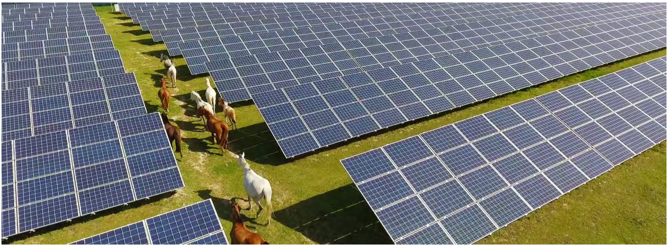
Fig. 59- PV plant owned by Finerge with 9.6 MWp installed in Coruche, Portugal. Source: Voltalia
